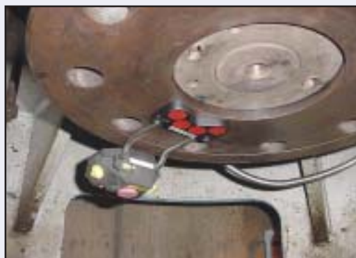
Photo 1. The laser emitter was installed on the motor shaft. This was done by attaching a magnetic bracket with offset support posts to the face of the rigid motor coupling.
