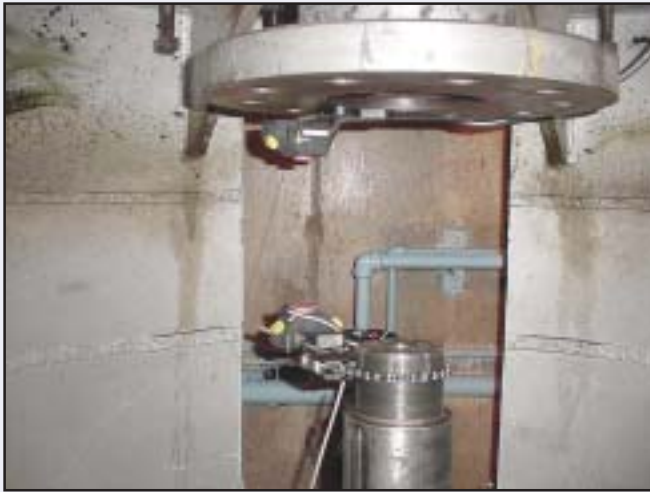
Photo 2. The receiver is mounted on the pump shaft using a standard chain bracket.
